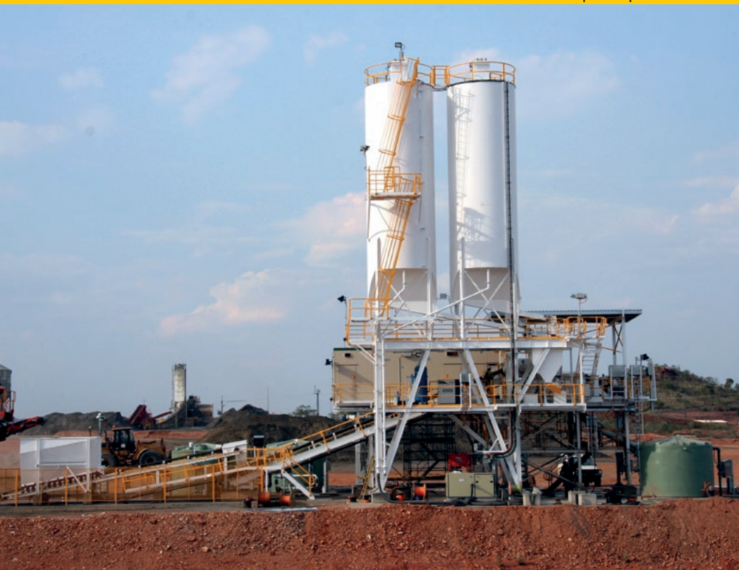
350 tonnes per hour static backfill paste plant
