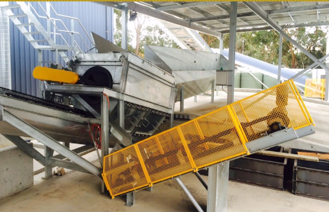
Reclaimer, truck wash out trough and conveyor
