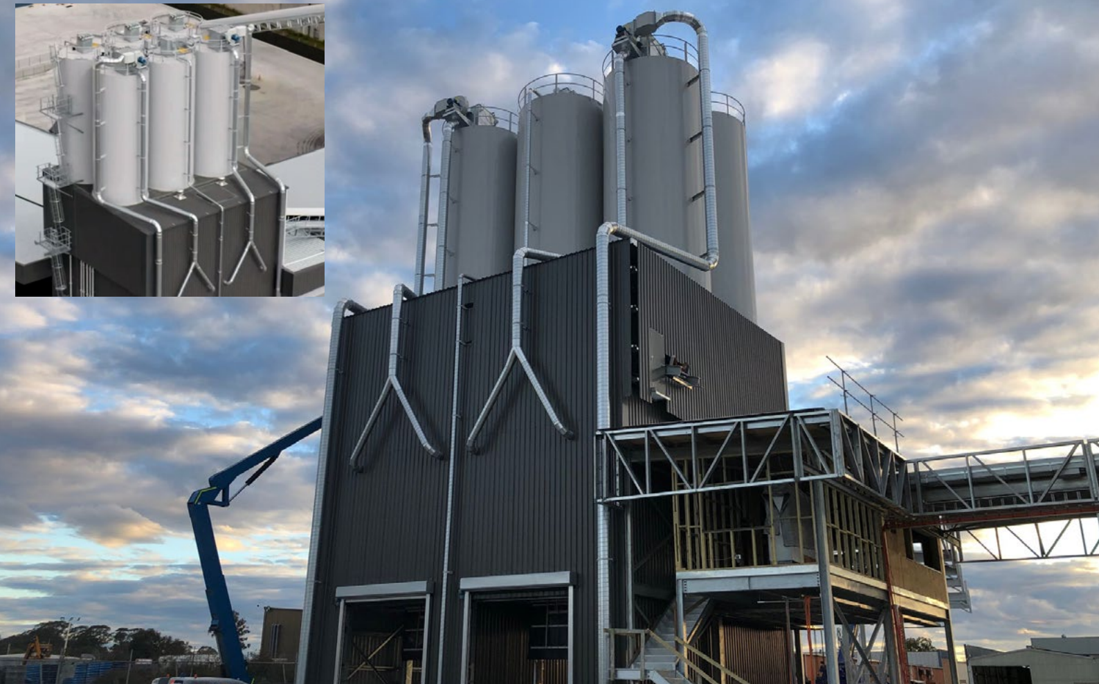
6 x 200T cement storage silos at concrete plant in New South Wales, Australia
