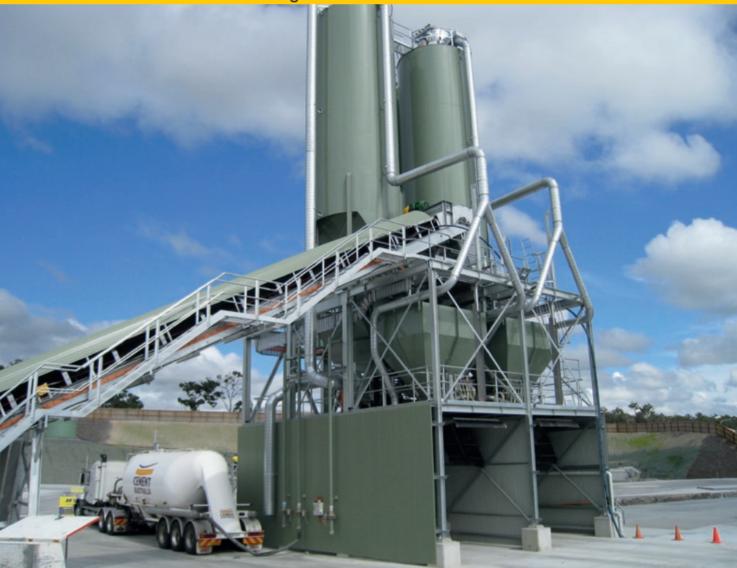
120T dual outlet cement silos feeding cement hoppers
