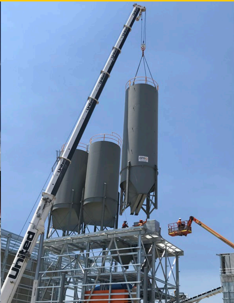
200T split cement storage silos
