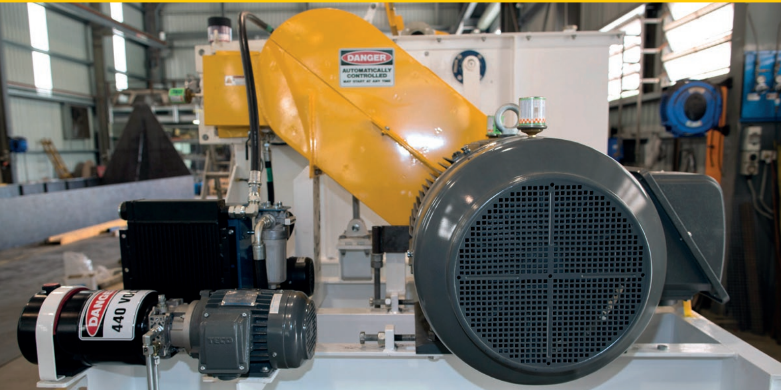
Hydraulic pump and drive assembly
