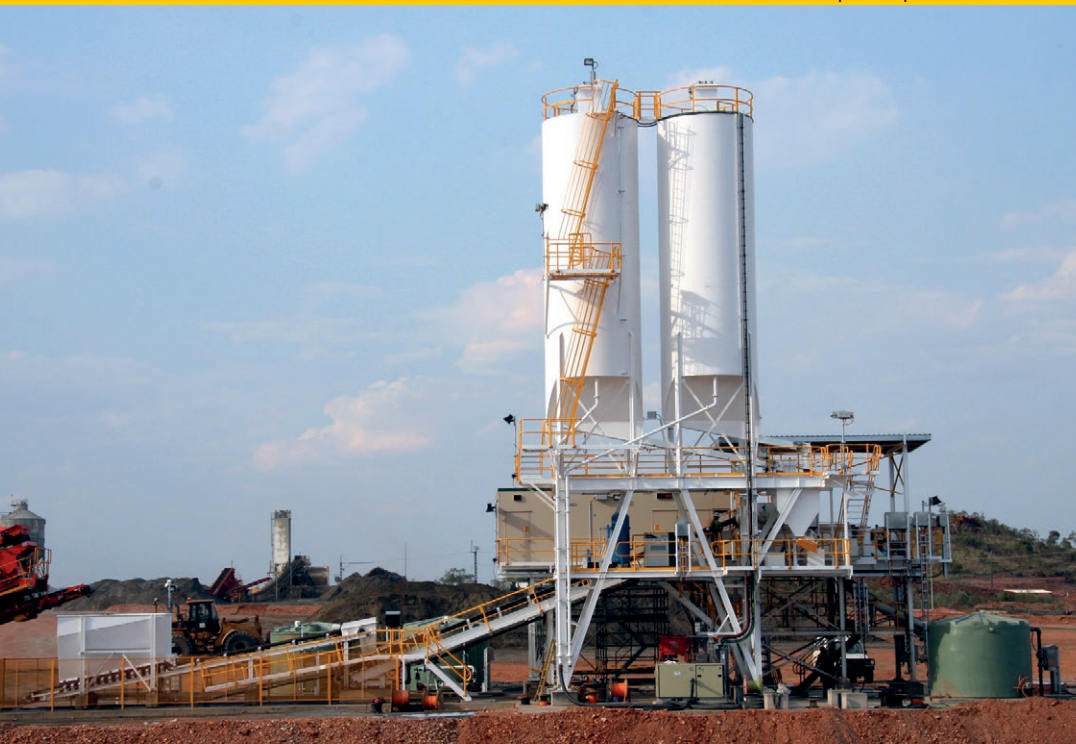
400Ton per hour static backfill paste plant
